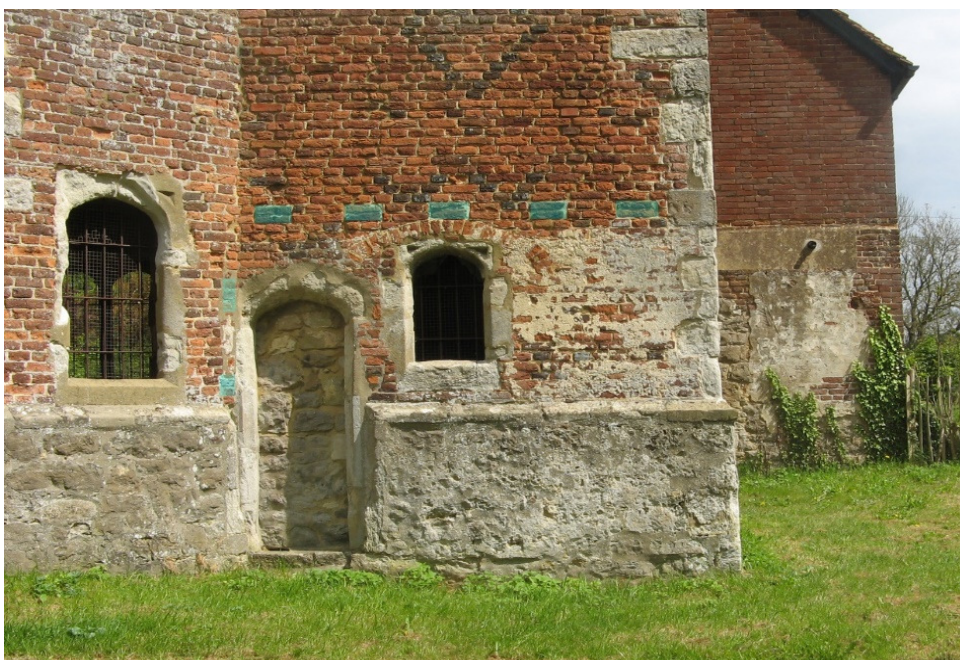
Fig 18 The south side of the garderobe tower showing blocked sockets for rafters, and probably rails of timber-framed wall, and internal plaster on the formerly external wall
