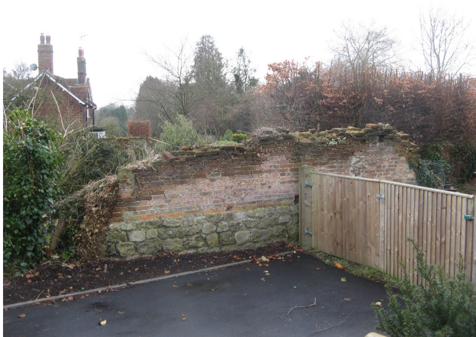
Fig 26 The remains of the north gable of the scheduled structure by the reservoir
