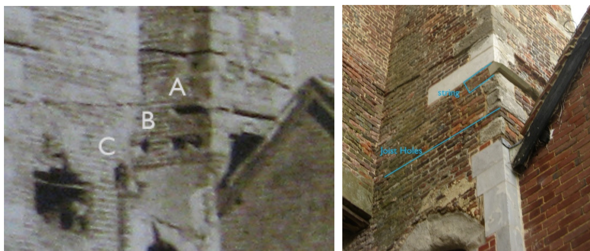
Fig 24 The north-west stair tower at second floor level in 1934 and 2017 showing (A) weathering course returning but now cut off; (B) gallery roof joist sockets now lost; (C – 1934 only) socket for bead of timber frame of west wall of the west gallery. Note extensive survival of internal plasterwork below joists 'B' in 1934; barely a fragment now remains
